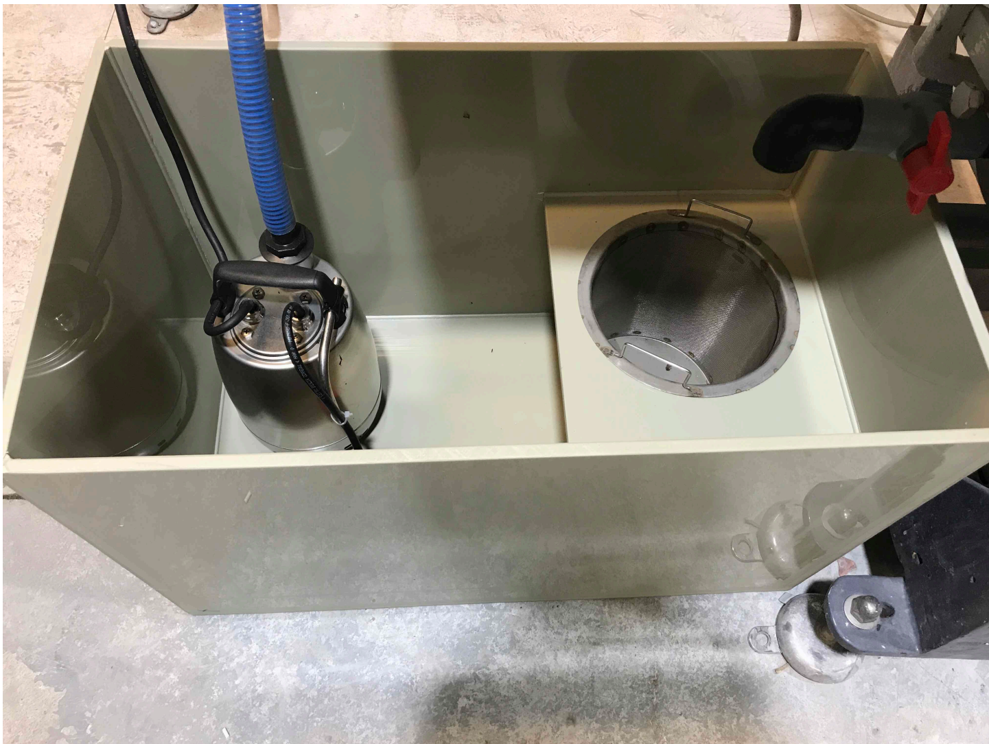
90 L. Buffer tank w/pump and filter basket
